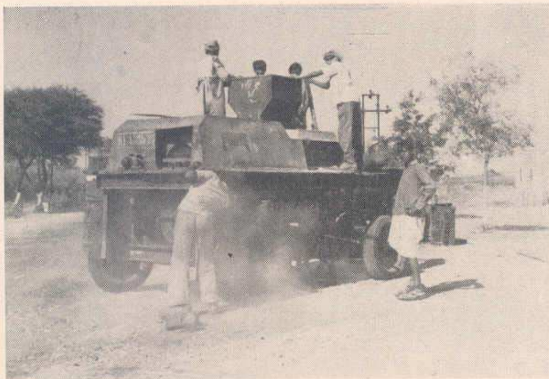
Photo 3. Cold mixing plant
